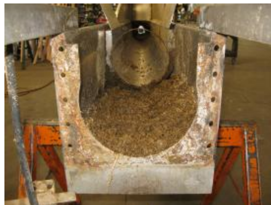
Fig 5 (screen removed to reveal plugged chamber)
